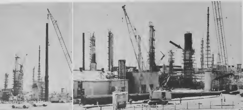
At left, the old section of the 83-ft high splitter lower before removal. At right, preparations are made to take down the furnace stack.
